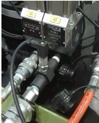
Figure 6.12 Test of the pressure sensor
