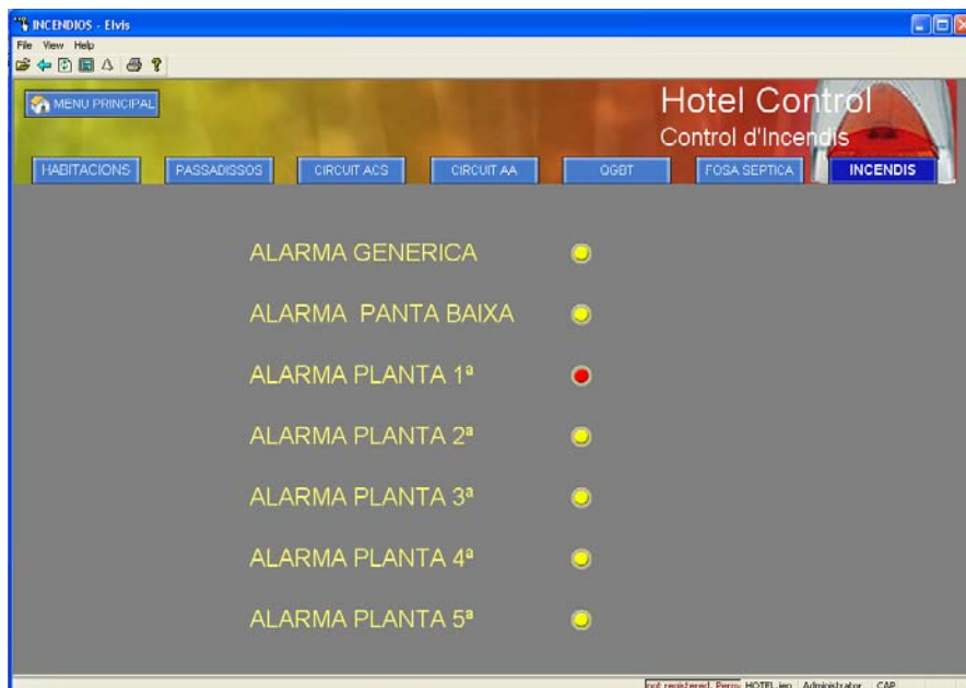
Figura 69: Control alarmes incendis
