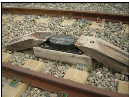
Figura 3.2.3.3 - Balisa ASFA (Font: Ferropedia - Article " ASFA ")
